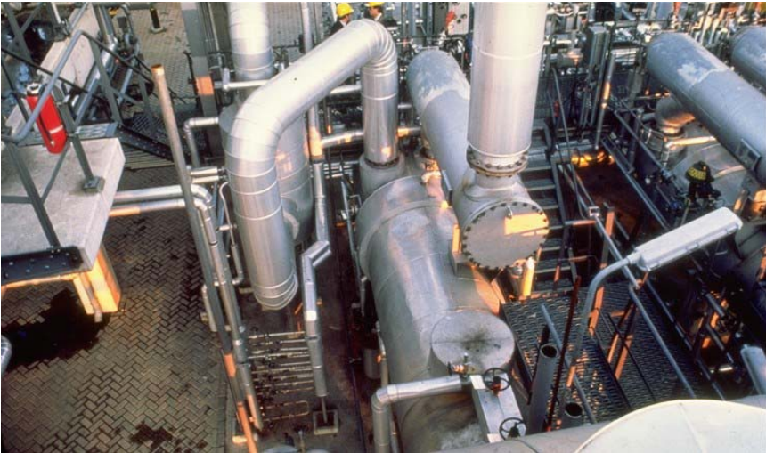
Air Preheater + Main Combustion Chamber
