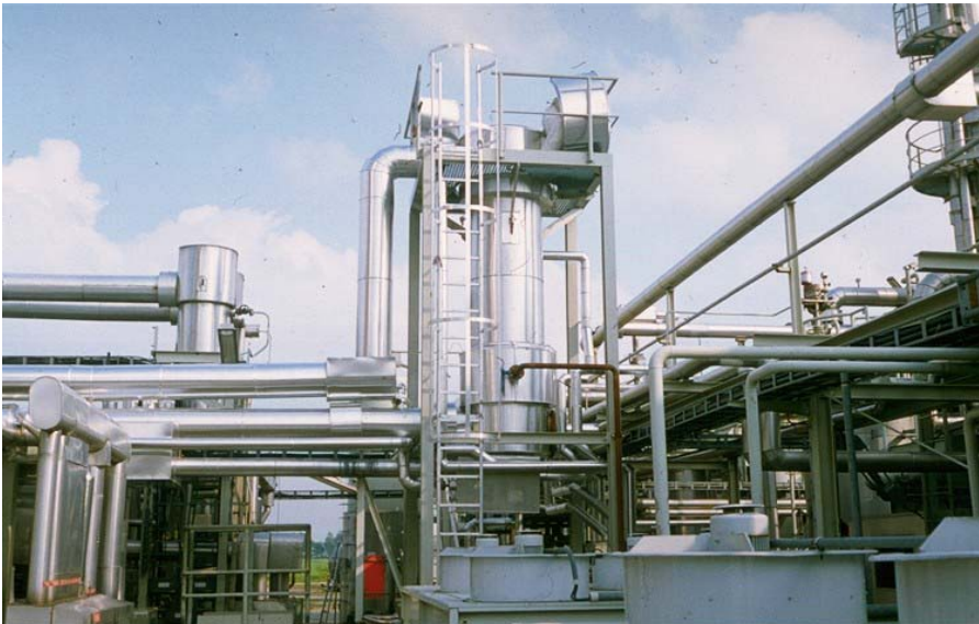
Project: Deep Cooler Client: Wintershall, Rutenbrock
